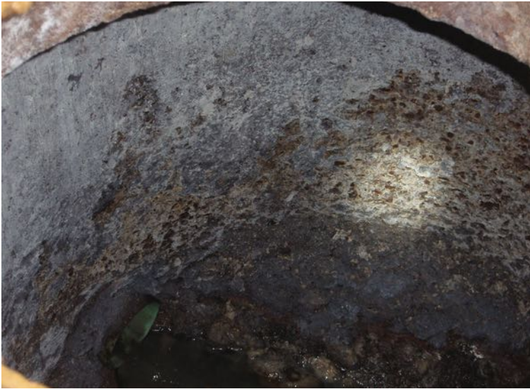
Corrosion of the concrete surface near the invert of a sewer manhole
