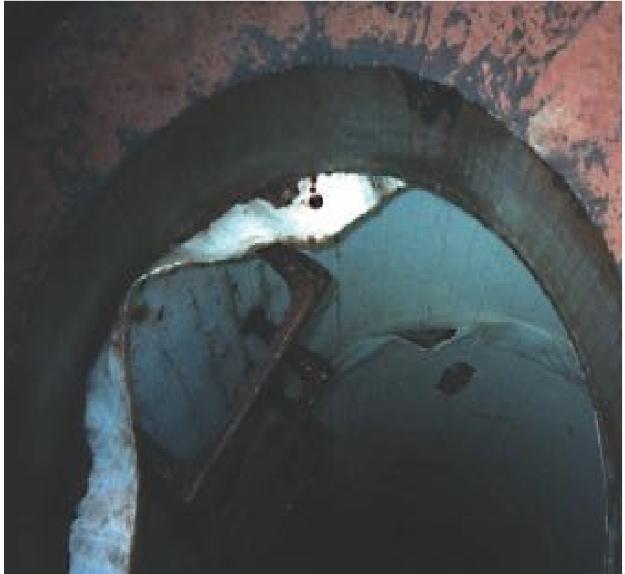
PVC liner in a manhole. This was not installed correctly. Already, the joint is exposed due to a poor weld. In the worst case, the liner will fall into the base and block the sewer line.
