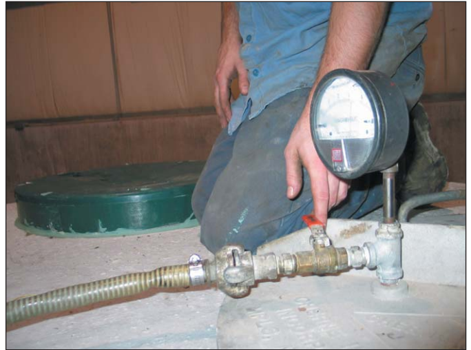
Concrete tanks can easily withstand vacuum testing to 4 inches of Hg, but polyethylene risers have trouble. Note the sucked down lid which continued to leak. The space between riser and concrete held after a bead of caulk.
