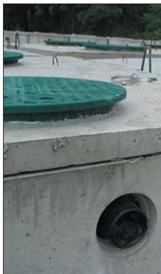
Watertight top-seam tanks at Rosenberry's, Shippensburg, PA. Clamps for the rubber seals are next to the risers. No rain water gets into the tanks. Contractors love them.
